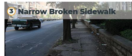
3 Narrow Broken Sidewalk The existing sidewalk today is in poor condition. With trees creating cracks in the sidewalk and a narrow walking space, this area can be uncomfortable for users.
