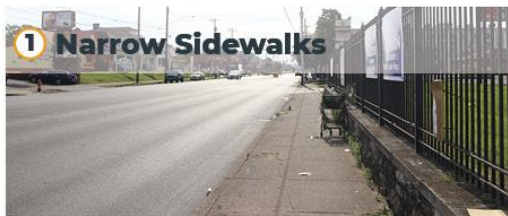
Existing sidewalks along the north side of the intersection are only 5' wide. This creates an uncomfortable walking experience for pedestrians.
